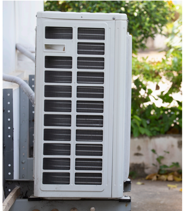
Air source heat pump
