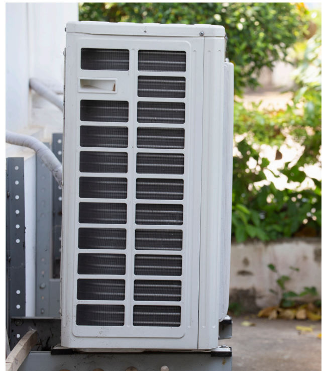
Air source heat pump
