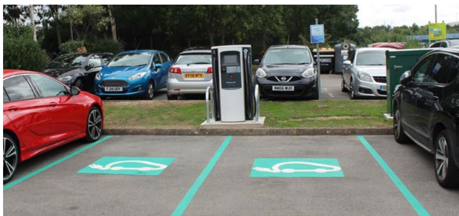
Figure 3 – A rapid chargepoint well-positioned within a car park
