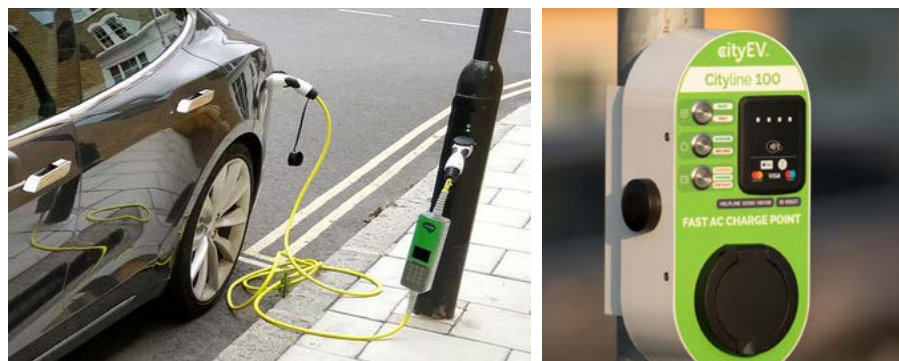
Figure 4 – Lamppost chargepoints of different designs
