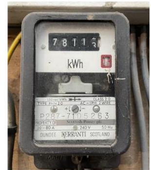
Site electricity meter
