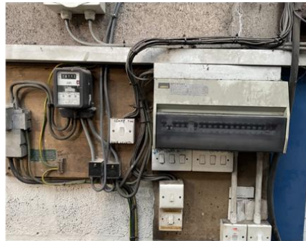
Internal master fuse, circuit breaker
